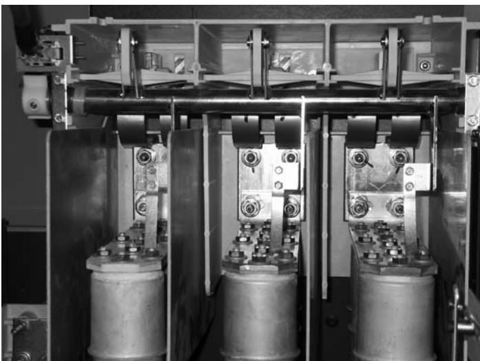
View of Isolation Switch Through Viewing Window
