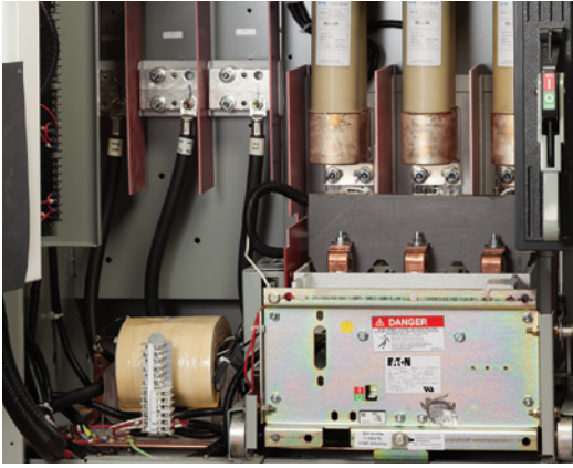
Ampgard XP3 Medium Voltage Starter with MV Door Open
