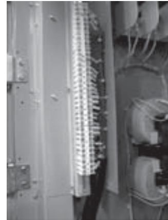
Figure 9. Low Voltage Terminal Blocks, Medium Voltage Door Open
