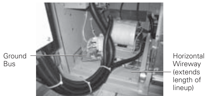
Figure 18. Horizontal Wireway and Ground Bus
