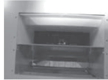
Figure 16. Medium Voltage Cable Conduit Area (View from Top Rear of Bus Compartment)
