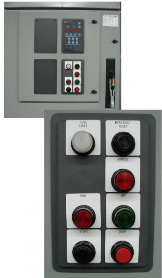
Figure 3. Low Voltage Components
