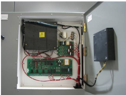
Figure 8. Control System Boards
