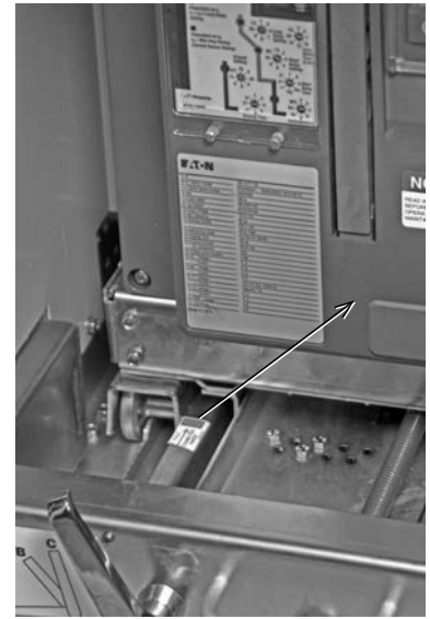
Circuit Breaker in Connected Position Indicator
