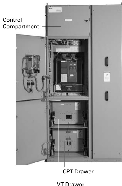
MEF Switchgear—Indoor Unit
