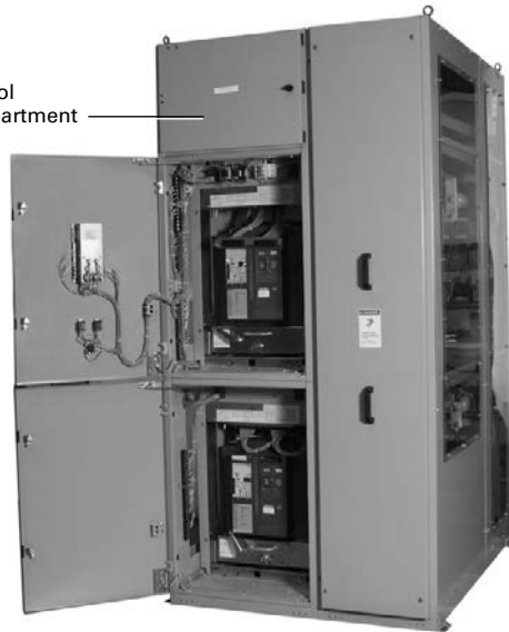
MEF Switchgear—Breaker Over Breaker and Adjacent Pull Section
