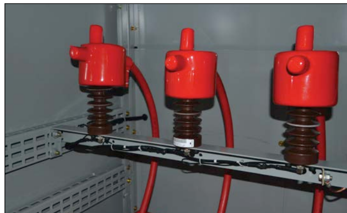
Figure 6.1-9. OVS Sensors Mounted in Cable Compartment
