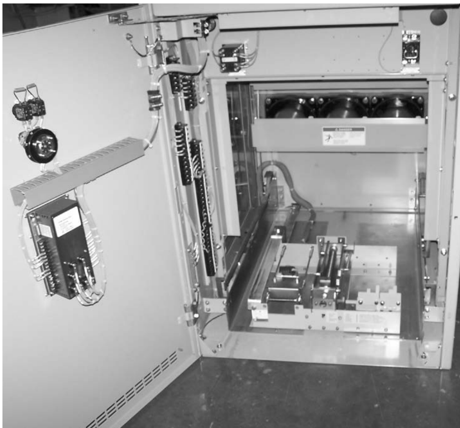
Roll-on-the-Floor Switchgear Compartment
