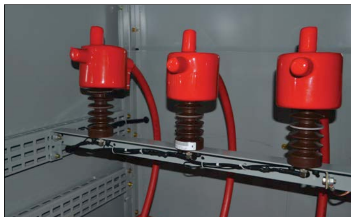
Figure 5.1-8. OVS Sensors Mounted in Cable Compartment
