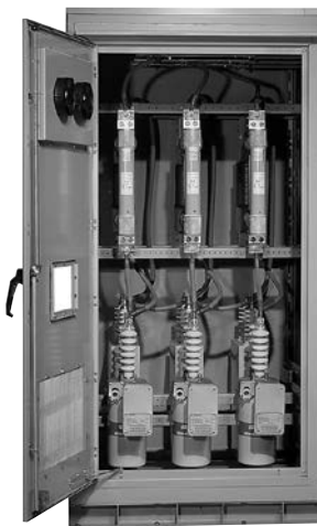
15 kV switched capacitor stage enclosure
