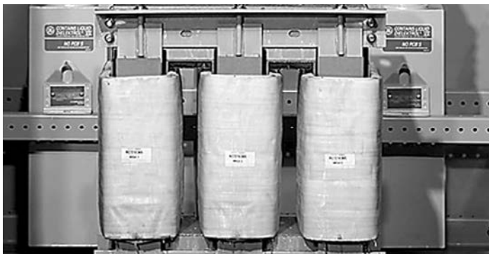
Reactors for detuned filter
