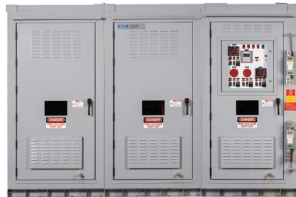
Medium-voltage AutoVAR with three vertical sections shown with the incoming section on the right hand side.
