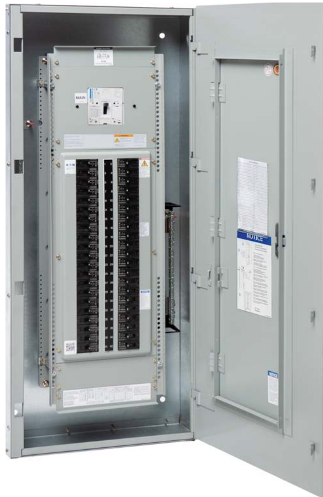
Trim Hanging on Surface Mounted Box
